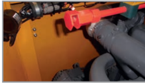
Fire Fighting System
